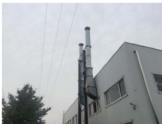
1#漆房及2#喷漆房排气筒
